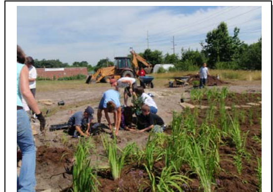
Rain gardens like this one planted with the help of volunteers in New Castle County, DE are one example of “green infrastructure.”
